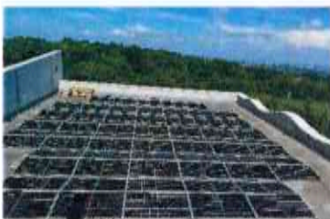
Sanatoria Klimkovice Klimkovice 702,45 kWp
