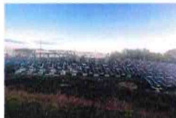
MS UTILITIES & SERVICES a.s., Bohumín 1,1 MWp
