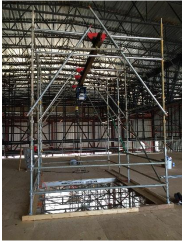
Figure 8a – Material Hoist
