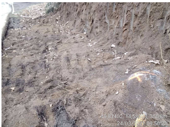
Obr.8 – balvan v km cca 0,360
