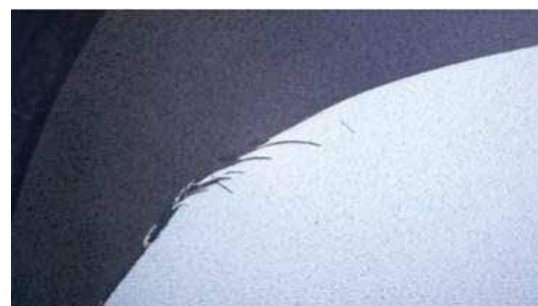
Rail Contact Fatigue (RCF) on Head Hardened Grooved Rail
