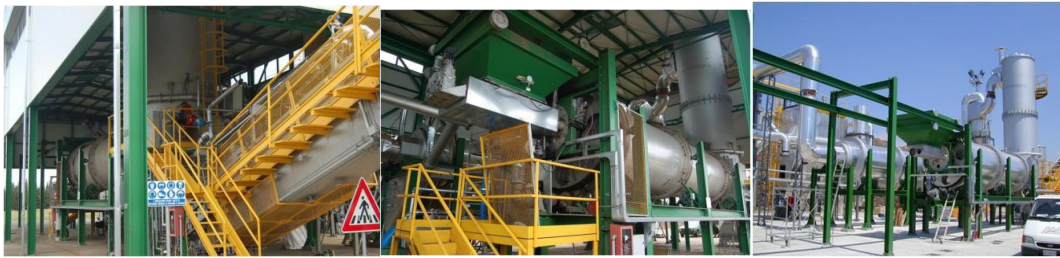
Example of industrial scaling-up carried out with CSM contribution (2 t/h plant for production of grit from ASR fine fraction)
