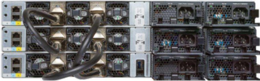
Figure 5. Cisco Catalyst 9300 Series switch stack units
