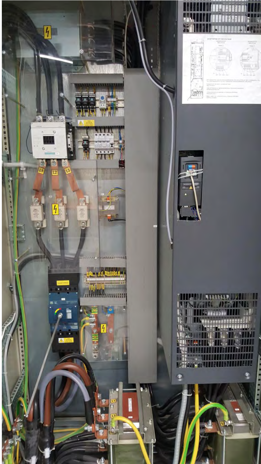
Figure 6.5.1 display of the frequency converter rack cabinet
