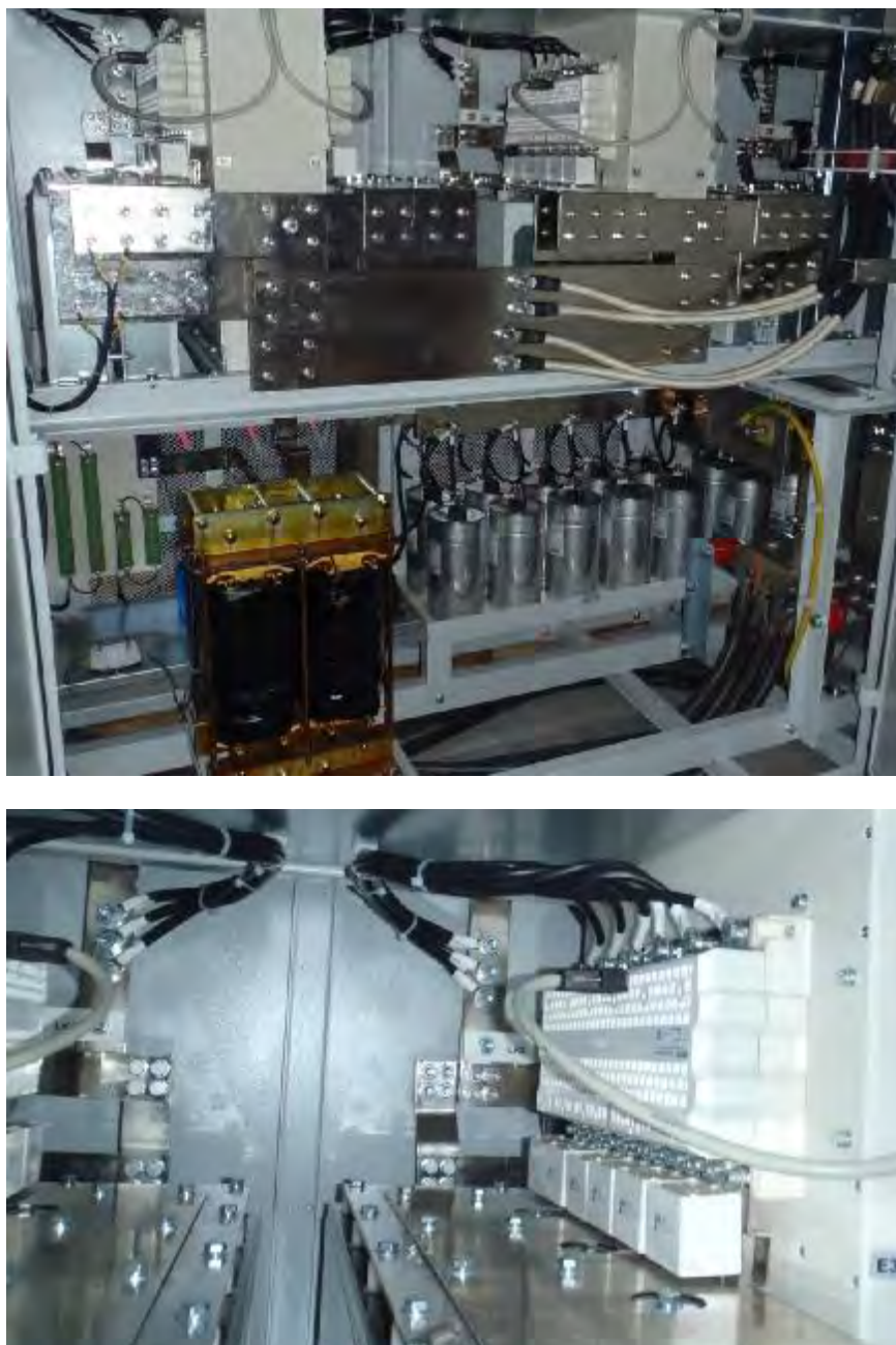
Figure 1. The IGBT air cooled converter using power modules manufactured by contractor.
